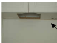
(Fig. 1) (Electrical power access)
